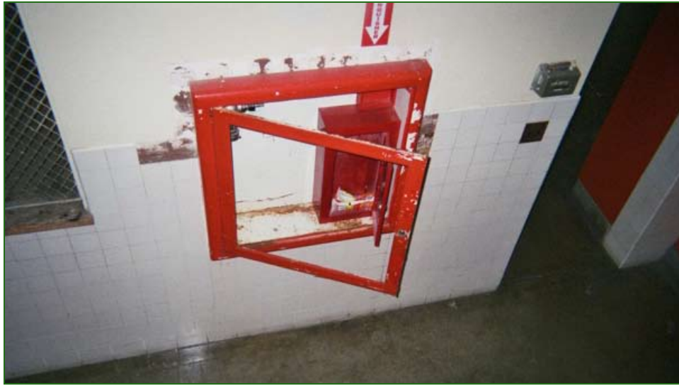
"This is a picture of where a fire extinguisher is supposed to be, but instead there is tagging and garbage. Also, instead of there being glass it is broken. That makes me feel unsafe..."
